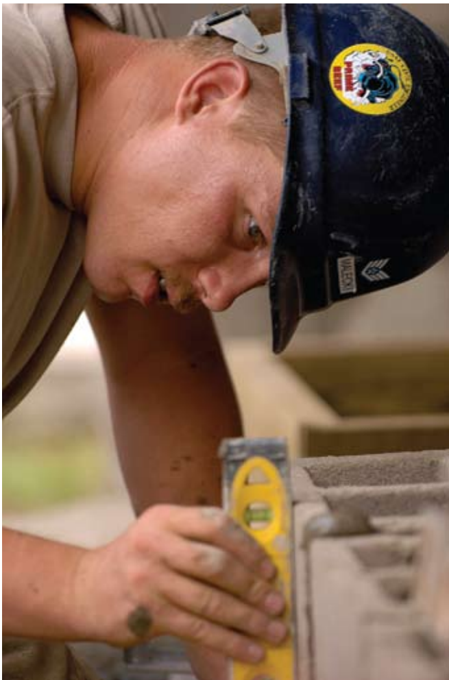
SSgt Arthur Malecki of the 5 CES, Minot, N.D., helps make repairs to The Best Hospital in West Demarara, Guyana. (U.S. Navy photo by MC Ernest Scott)
